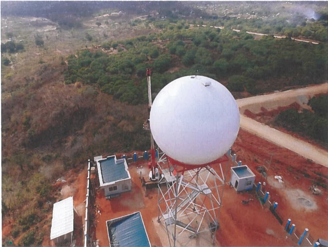
Fig.5: Weather Radar station at Mtwara
