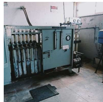
Fig. 5: (very) old/defunct H 2 generator at the UAS sounding facility, Espargos, Ilha do Sal
