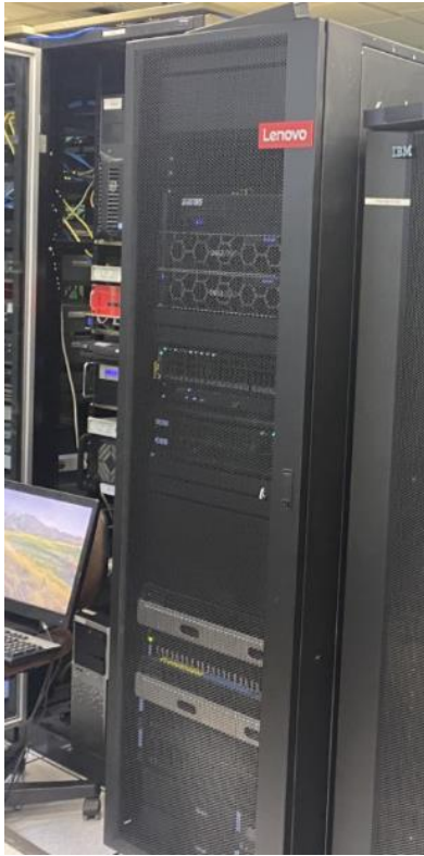
Figure 11 - Recently installed HPC server (Photo: authors)
